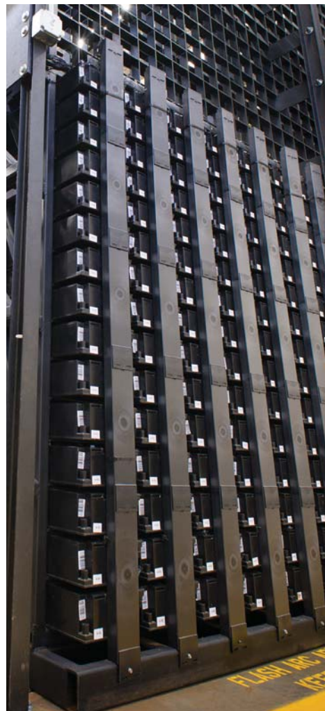
8 MWh of PowerCells in Double High Racks
